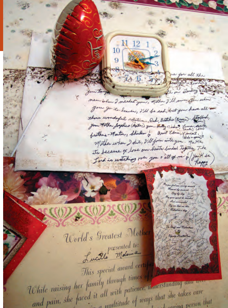
The wall of a resident’s bedroom shows where the water line reached, midway to the clock, at St. Rita’s Nursing Home where more than 30 dead bodies were found nearly two weeks after Hurricane Katrina.
